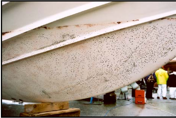
Fig 14. A poorly prepared laminate.
