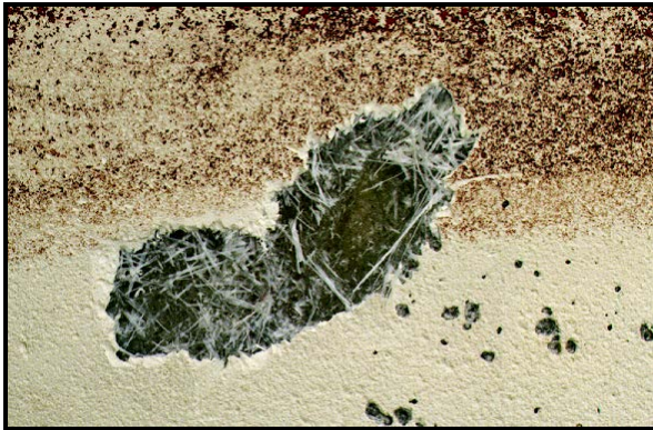
Fig 16. Unbound fibre behind a yacht's gelcoat.
