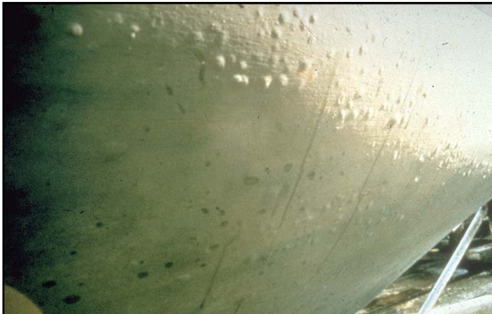
Fig 11. Blistering like this takes many years to develop, and will not be cured by any amount of heating or de-humidification. The HotVac system has proved very successful for treating ‘problem’ boats, but peeling, blasting and thorough fresh water washing remain an essential part of the process.
