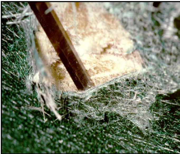
Fig 10. This poorly consolidated laminate had very little adhesion between layers of reinforcement, and was suffering from loss of mechanical strength.
